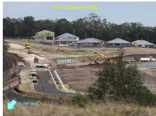
Figure 5. Construction activities were taking place ~365 m from a White-bellied Sea-Eagle nest at Fletcher on 1 August 2016.
