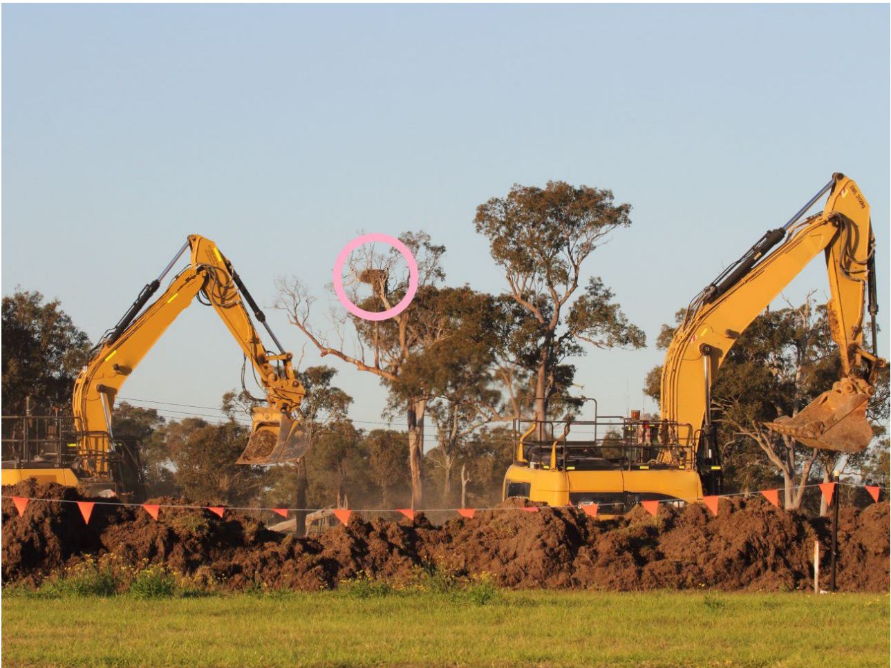
Figure 6. Two excavators were being driven <100 m from an active White-bellied Sea-Eagle nest (see Figure 2 ) at Chisholm on 18 August 2016.
